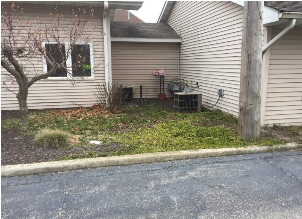
Photo 15: Air conditioning units on ground and rooftop
