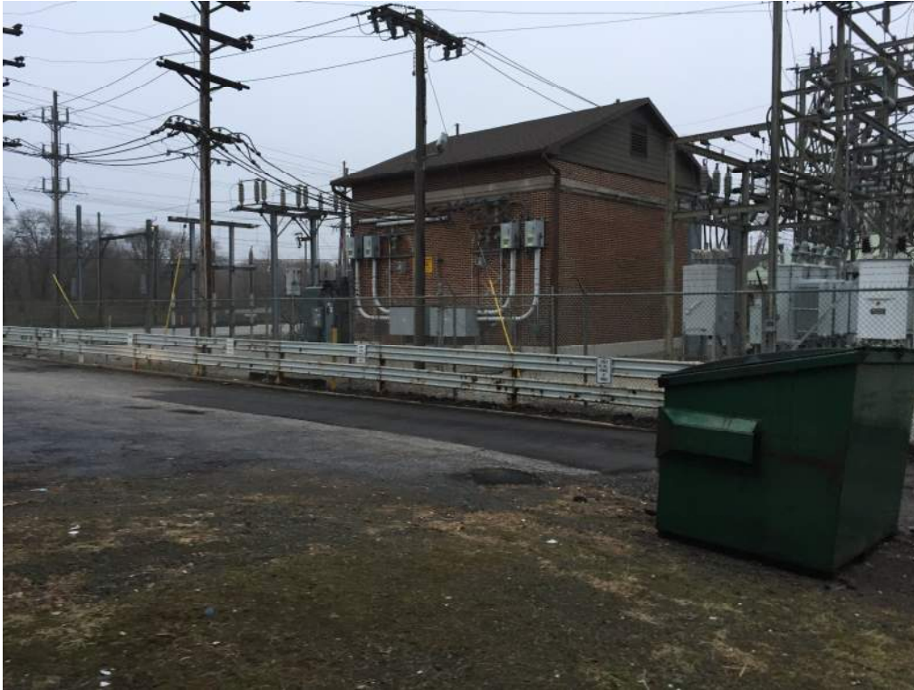
Photo 13: Electric substation on northwest adjoining property. Contains pad mounted transformers with slight rust staining on some transformers
