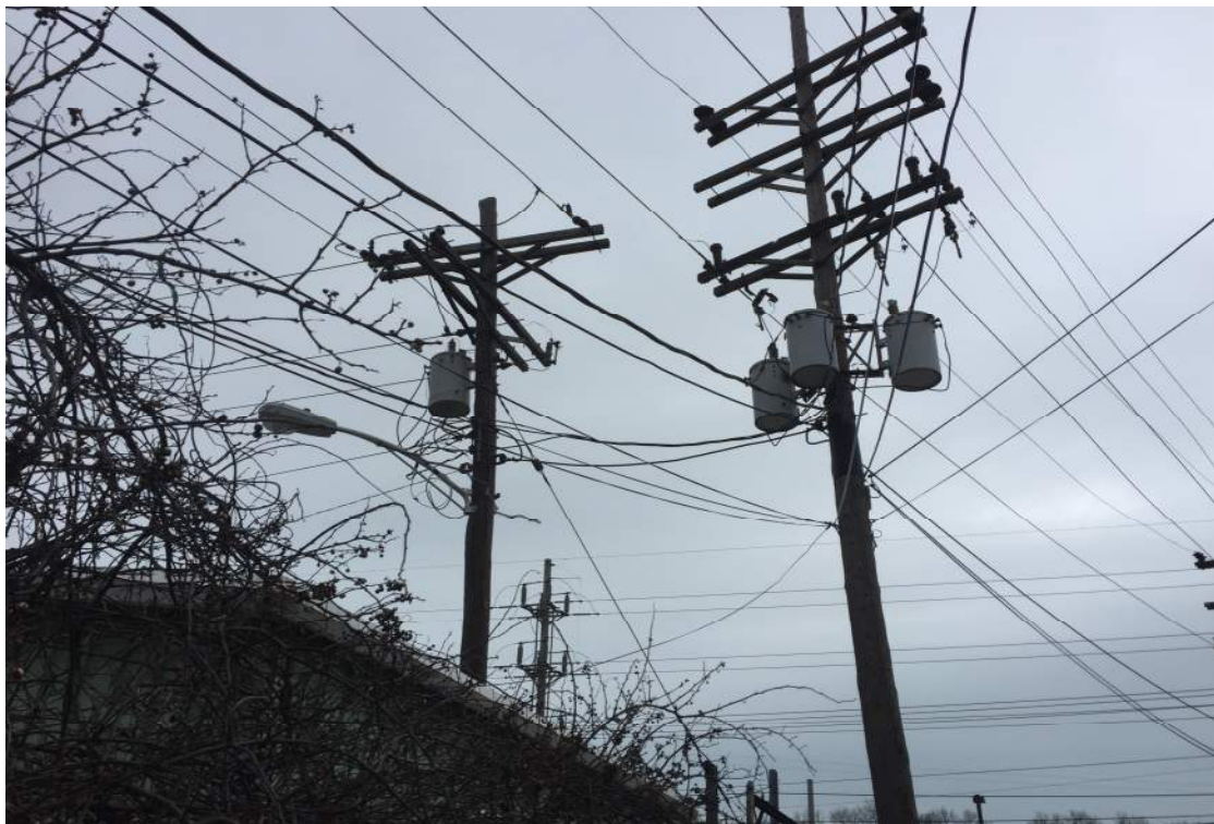
Photo 12: Four pole mounted transformers on northwest adjacent property
